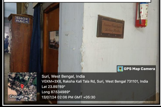
Fire Extinguisher Facility Seminar Hall
