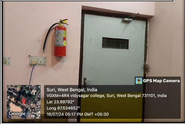
Fire Extinguisher Facility Language Lab
