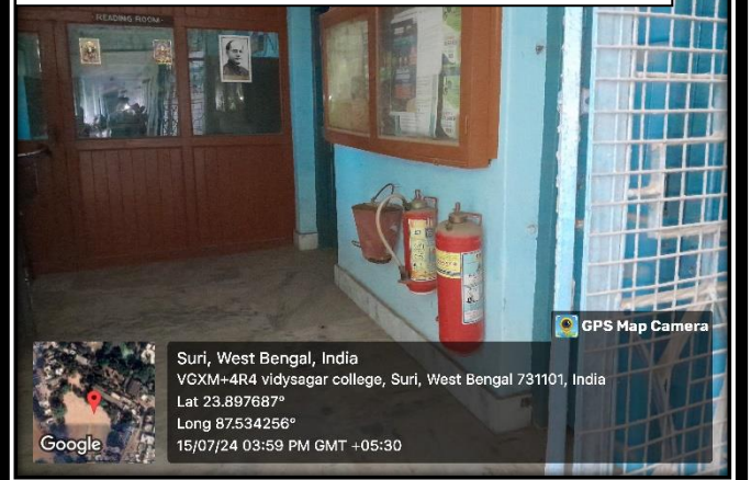
Fire Extinguisher Facility Day Library
